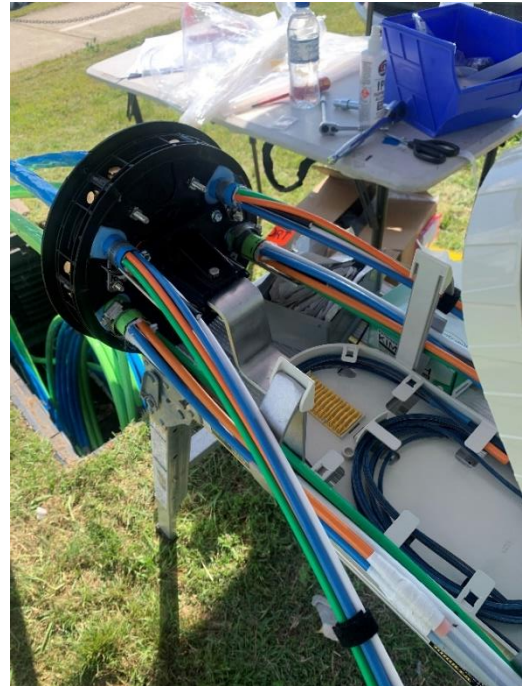
Figure 14 - View of the ribbons looped in the first tray and the other tubes ready for termination
