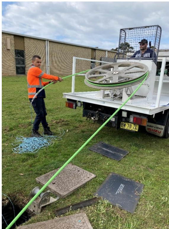
Figure 3 - Haulers bringing the flat ribbon cable out of the first pit (P6)
