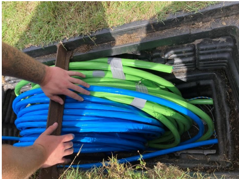
Figure 9 – P8 pit filled with cable coils after hauling. 15 + 25m of FlexRibbon™ cable was coiled with 15 + 15m of flat ribbon cable
