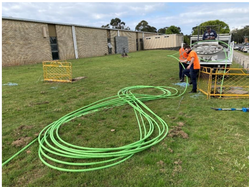
Figure 8 - Figure 8 lay up of flat ribbon cable as exiting from the first pit (P6)
