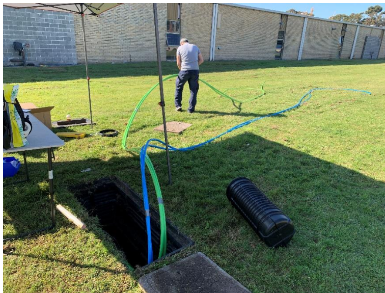
Figure 17 – Splicer working with the flat ribbon cable to cut it to the correct length
