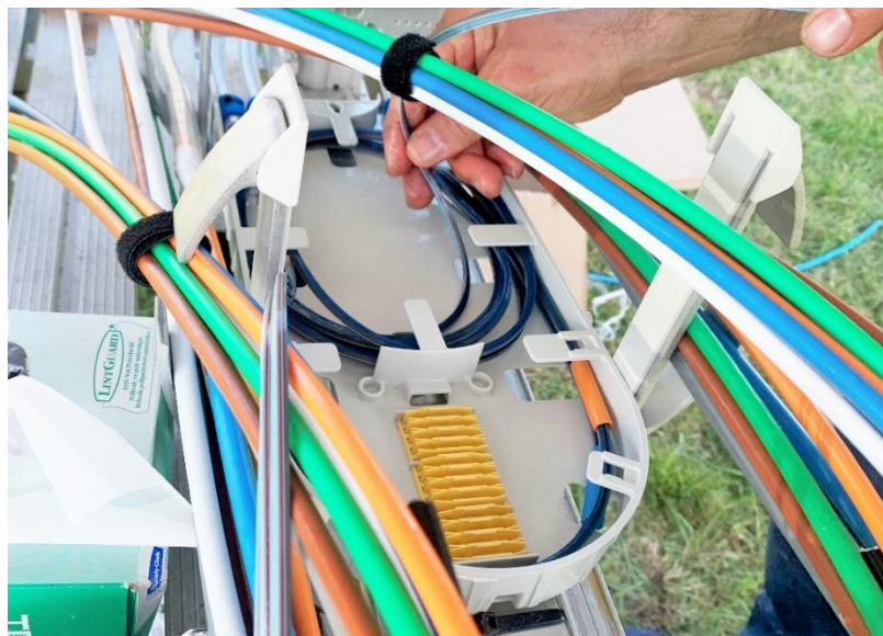
Figure 18 - Flat ribbons being looped around the fibre tray. Care was taken so that the ribbons were collectively looped around the tray on their preferential axis
