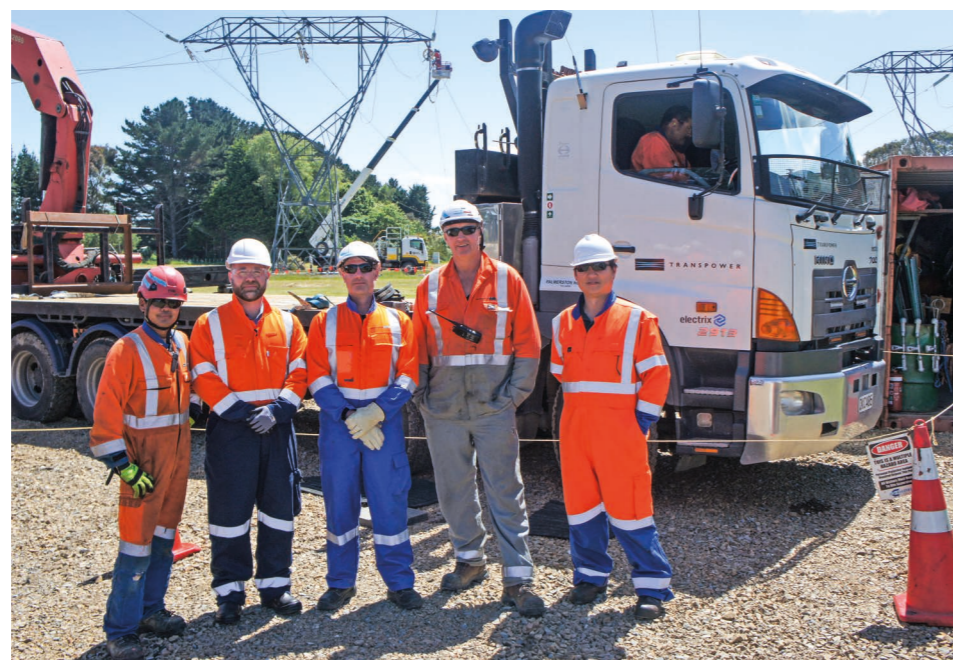
Teams from Prysmian and Transpower are working closely together to produce long-lasting line upgrades
